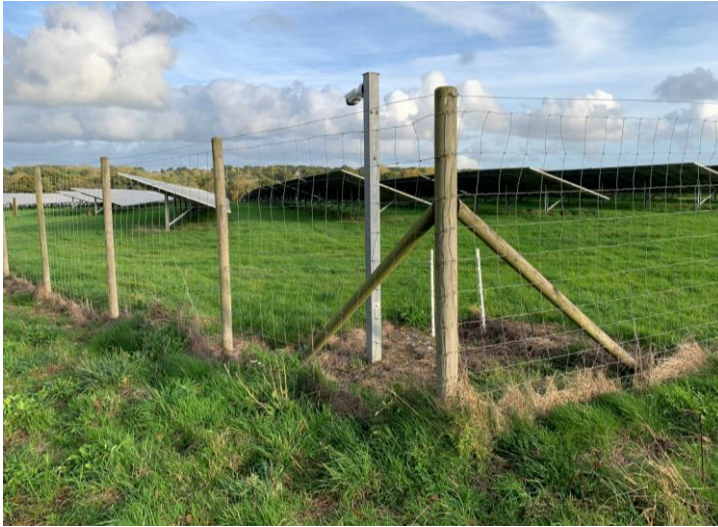
Photos 24 and 25: Typical CCTV Poles and Fencing
