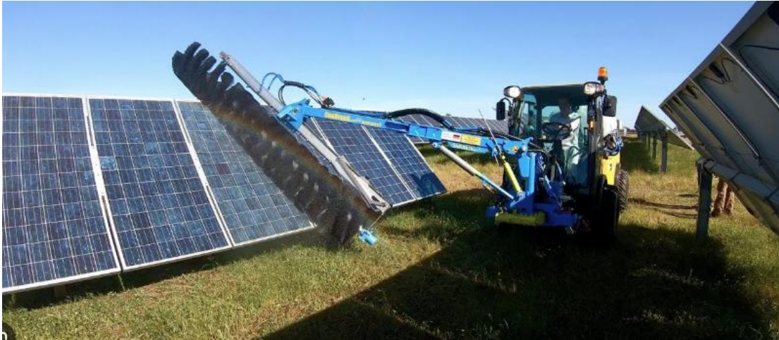
Photo 27: Cleaning of Solar Arrays
