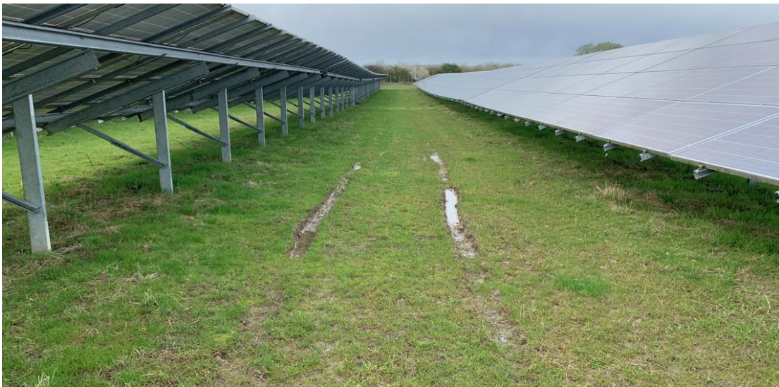
Photo 28: Ruts Caused by Vehicles
